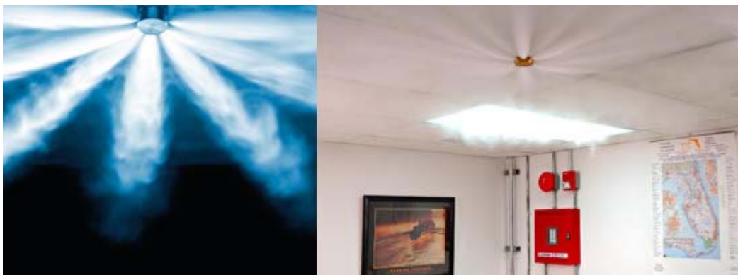
Figure 3: Example of Clean Agent System Discharge ( http://www.arafire.com.au/fire-suppression-systems.htm )
